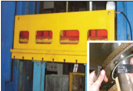
Main hot forming press and close up of damaged seals (size - 230 mm bore).
